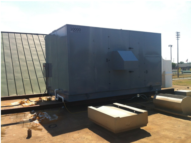
PrecisionDRY-ICE 10000 installed on the arena roof, July 2012.
