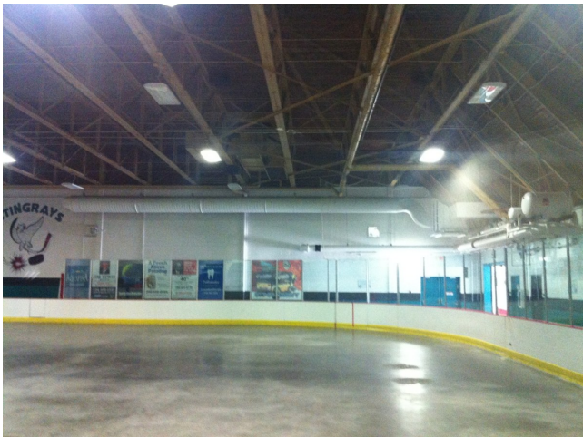
Conditioned supply and return ductwork serving the ice sheet and spectator areas.
